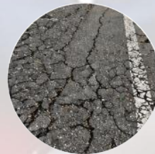
Distressed dense graded
