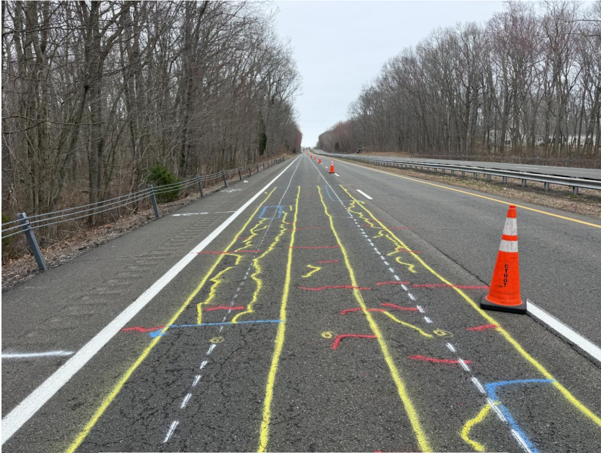
Field Labeled Crack Map
