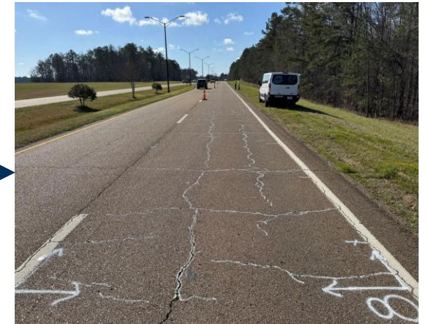
Real-world Crack (Ground Reference)
