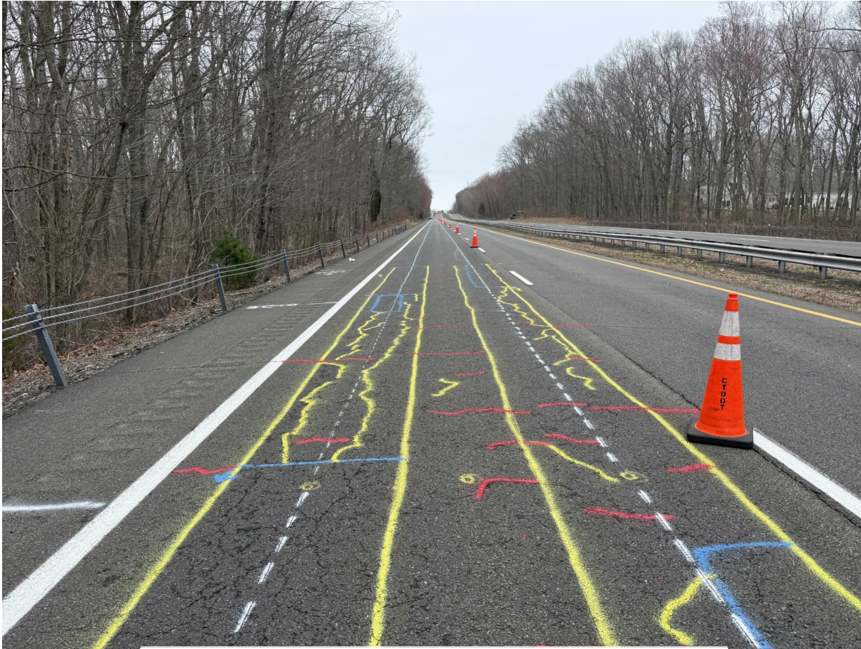
Field Labeled Crack Map
