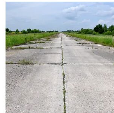
Joint Sealant Failure
