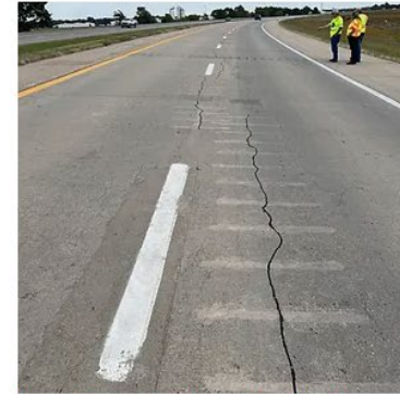
Low-Severity Longitudinal Cracks or Joints
