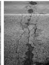
▲ Water enters unsealed cracks softening pavement and causing secondary cracks.
