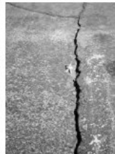
▲ Open crack — 1/2" or more in width.
