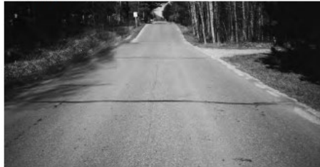
▼ Widely spaced, well-sealed cracks.
