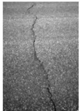
▲ Tight cracks less than 1/4" in width.
