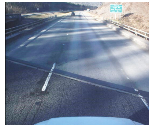
Low Texture/Aggregate Loss Caused by Concrete Bridge
