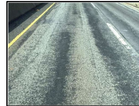
Severity Level 3 Loss of substantial portion of surface layer (>1/2 depth)
