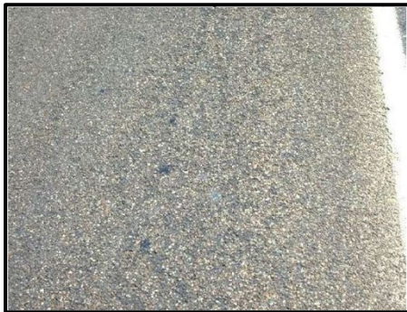
Severity Level 1 Loss of substantial number of stones
